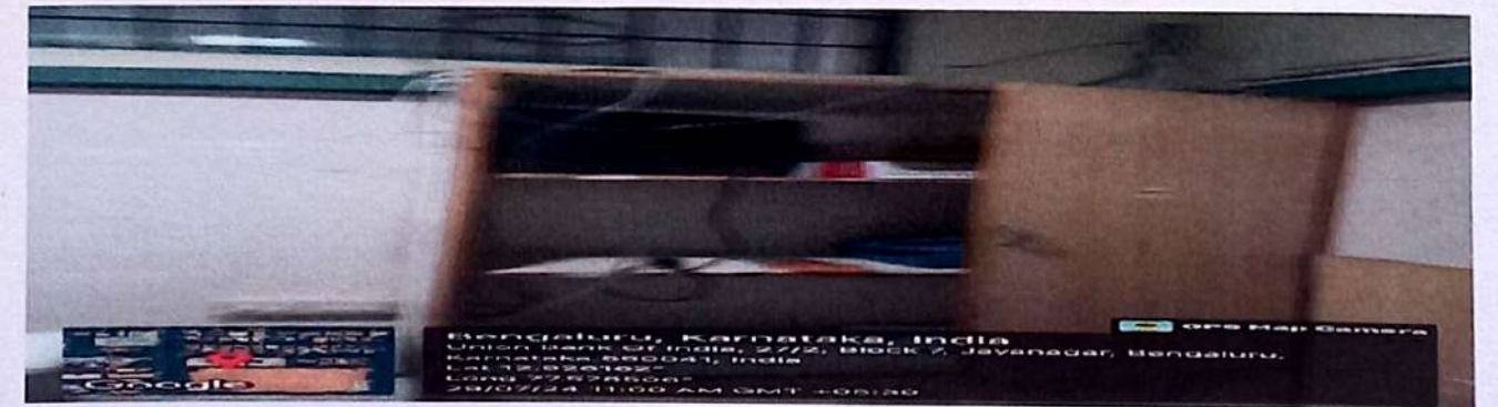
Wi-Fi Access Router and Network Devices
